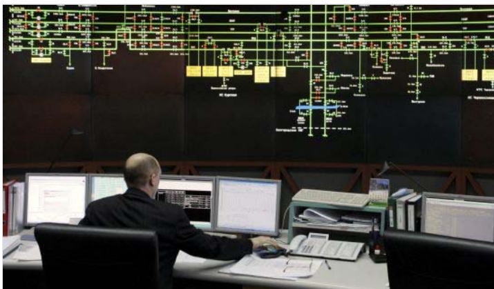
The control room at the headquarters of Gazprom, the Russian natural gas monopoly. (Misha Japaridze/The Associated Press)
